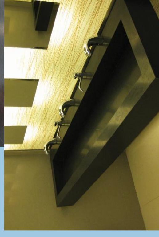
Automatic water tap sensors
