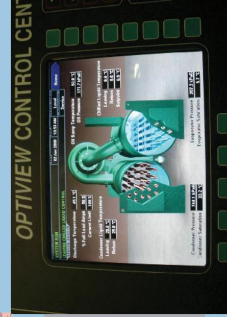
Variable speed drive and energy efficient chillers
