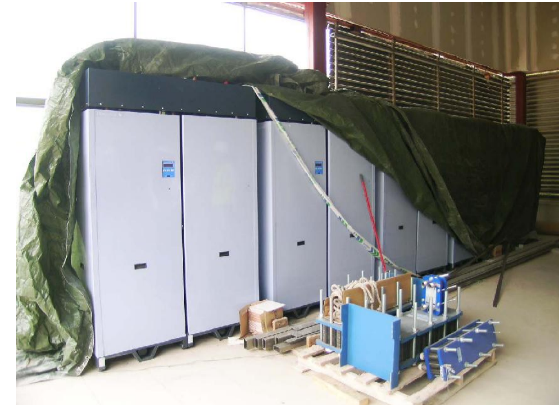
Absorption chiller room
