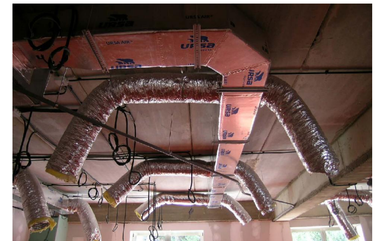
Handling units floor for latent cooling
